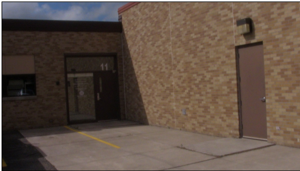
Figure 4.38 Another parking space potentially blocking adjoining doors
