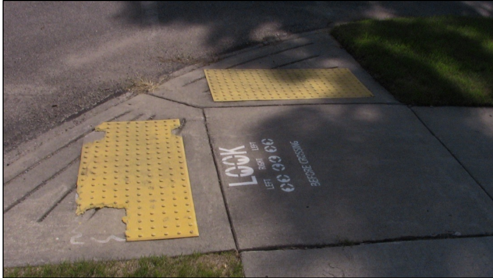
Figure 4.31 Damaged truncated domes
