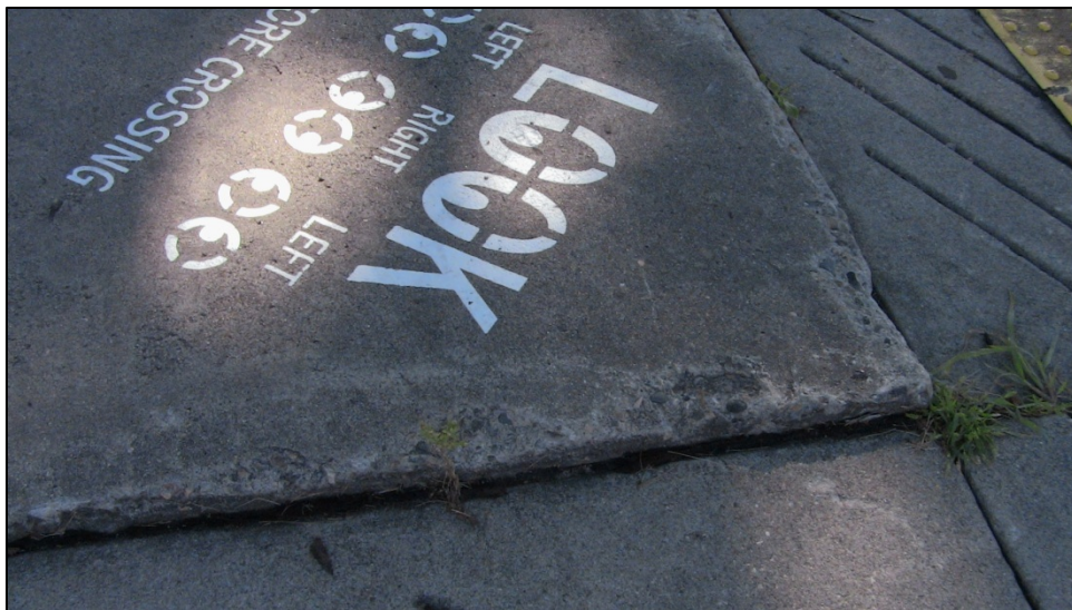
Figure 4.30 Faulting near crosswalk at the intersection of S 20 th St and 5 th Ave N
