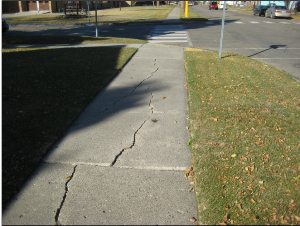
Figure 4.29 Longitudinal cracking in sidewalk slabs along S 20 th St
