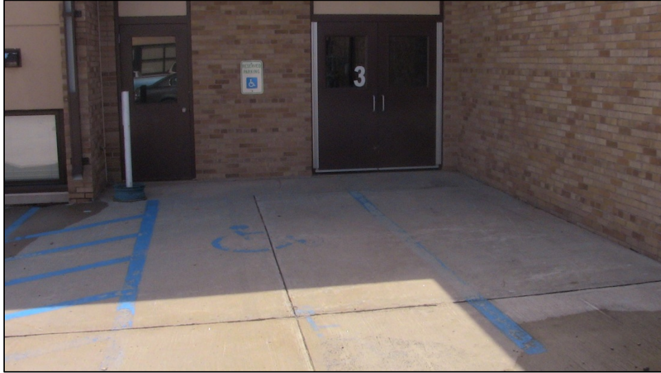
Figure 4.37 Accessible parking space blocking two doors in the north-east parking lot
