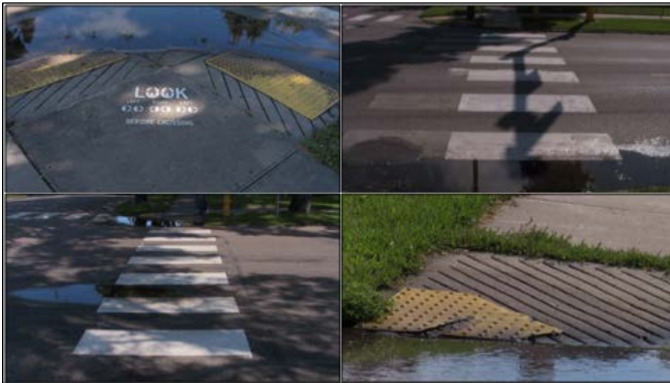
Figure 4.32 Poor drainage conditions and damaged truncated domes at S 20 th St and 5 th Ave N
