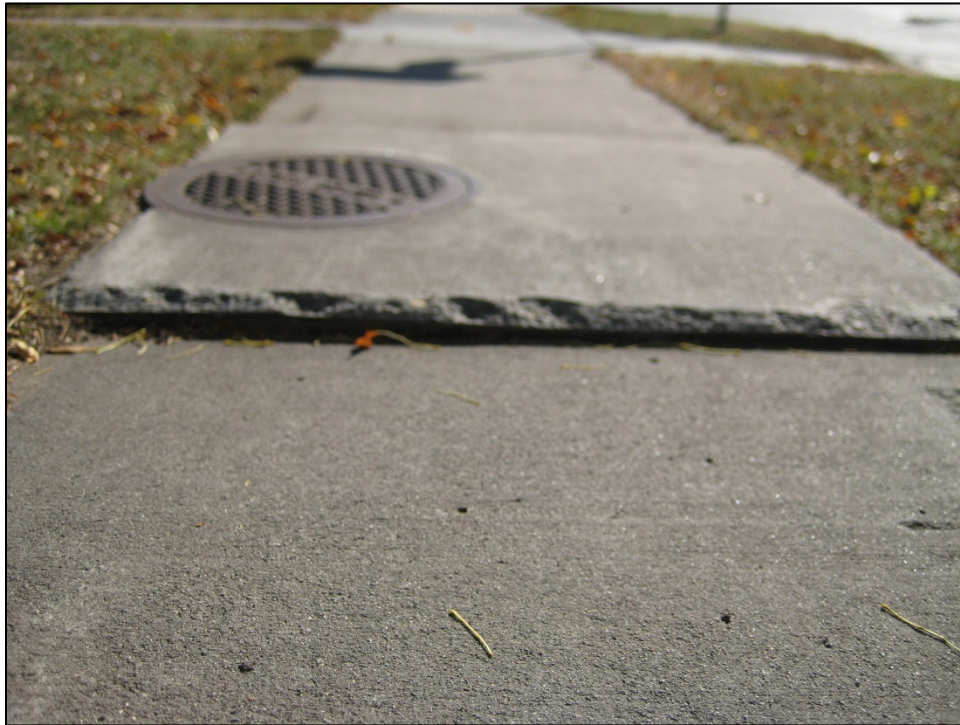
Figure 4.19 Faulted slab in sidewalk on the west side of the school
